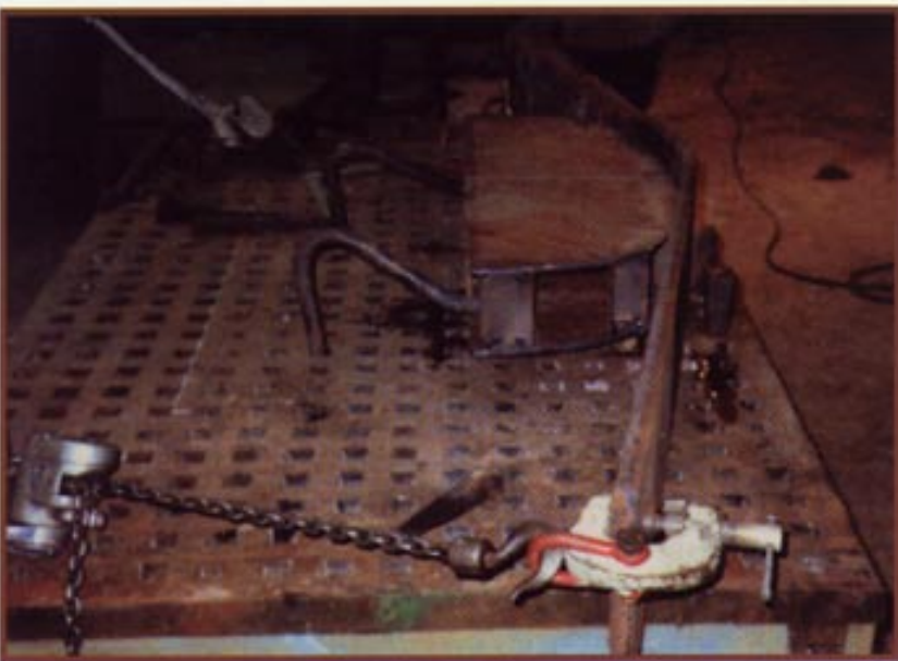
Figure 2 Tapered drift pins, gooseneck hold-down dogs, and two chain falls are used on this platen for bending.
